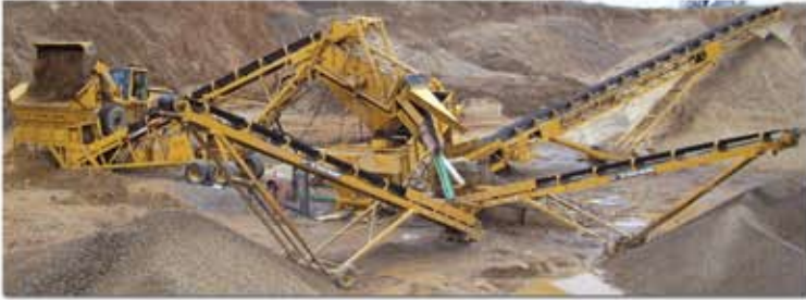
The Developer wash plant shown above has a 5' x 10" (1.5m x 3m) triple deck screen with spray bars, 44" (1.1m) sand screw, one 80' (24.4m) and two 40' (12.2m) radial stacking conveyors processing four sizes of washed aggregates
